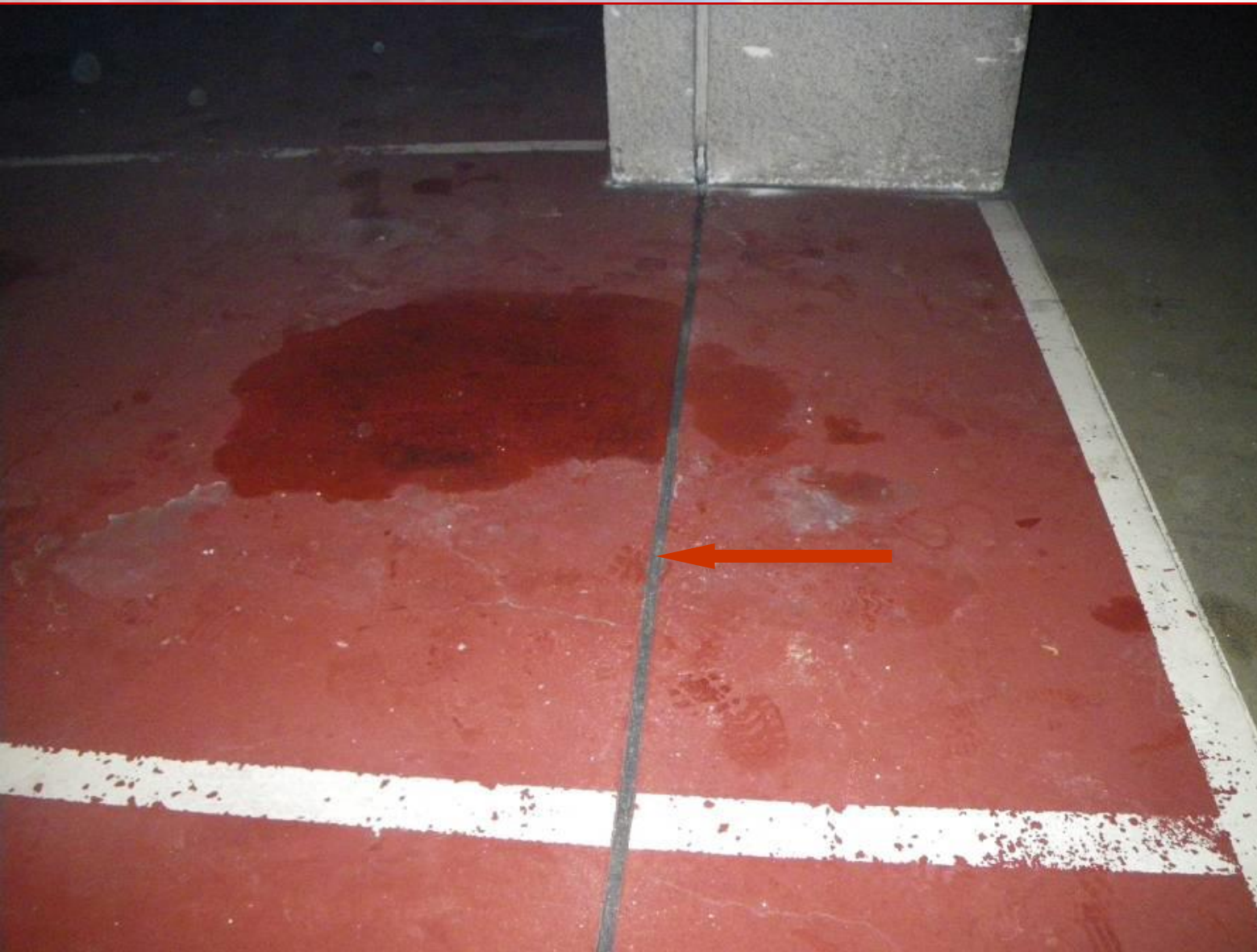
Joint de dilatation amianté (parking)
